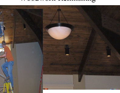
1 of 4 New Ceiling Lights
